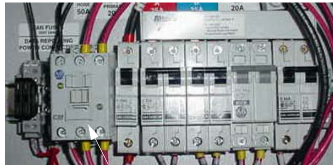
C30 Contactor Assembly Installed
